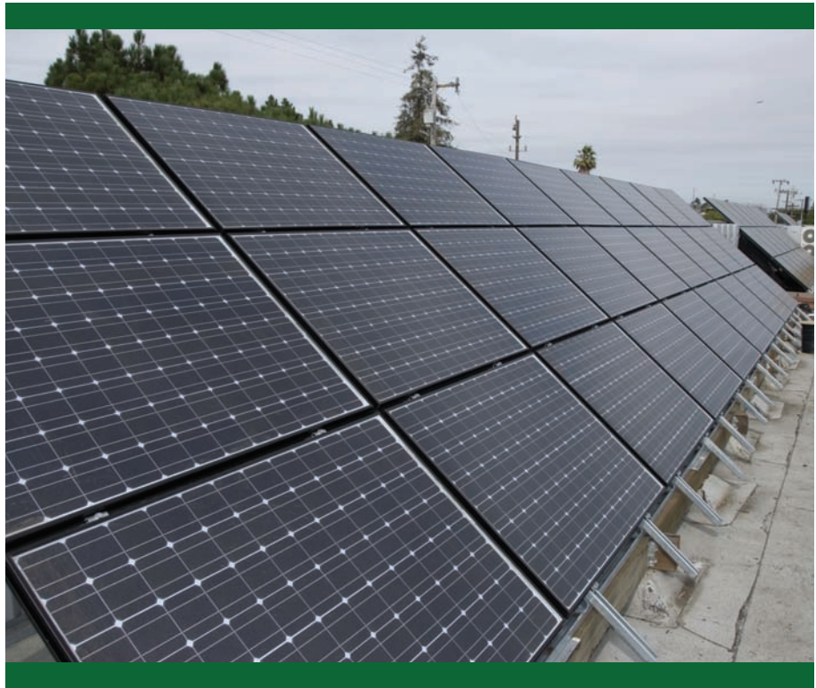
Barker Blue Digital Imaging, San Mateo, Calif., has gone green in a major way by installing a solar array on its roof. The array provides a majority of the shop's electricity needs.
